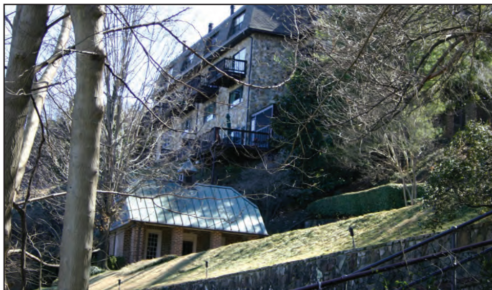
The landscape slopes down toward the Tennessee River in the back of these structures.
