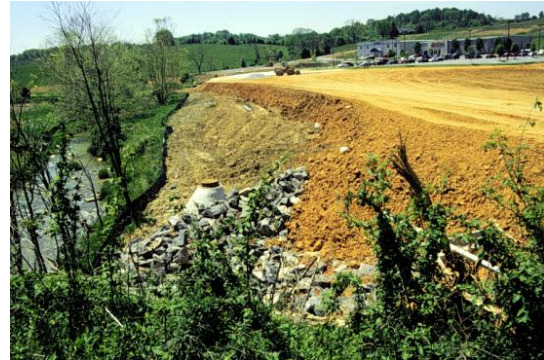
Figure 5.2.1.1-1. Clearing and grading a hilltop removes the ecosystem services inherent in undisturbed soils and vegetative cover.
