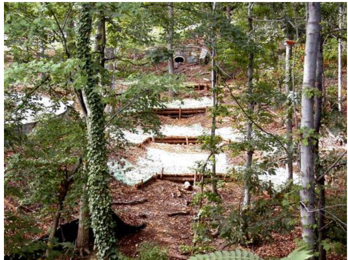
5.2.1.2-9. Check dams below outlet on steep slopes.
