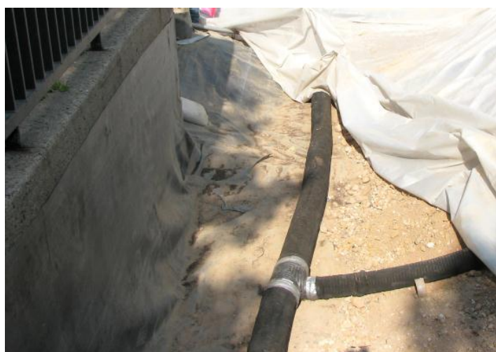
Figure 5.3.3-6. Impervious liners can be used to prevent lateral movement of water beneath standard pavement.
