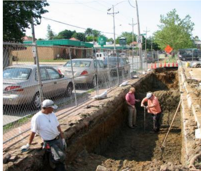
Figure 5.3.3-13. The bottom of an infiltration trench is level and uncompacted. The design engineer should observe conditions before the trench material is placed.
