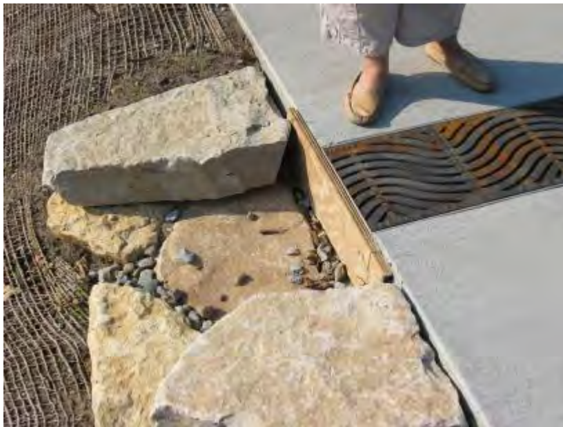
Figure 5.3.4-20. A trench drain outlet is closed to prevent sediment-laden water from entering the bioretention area until site stabilization occurs.
