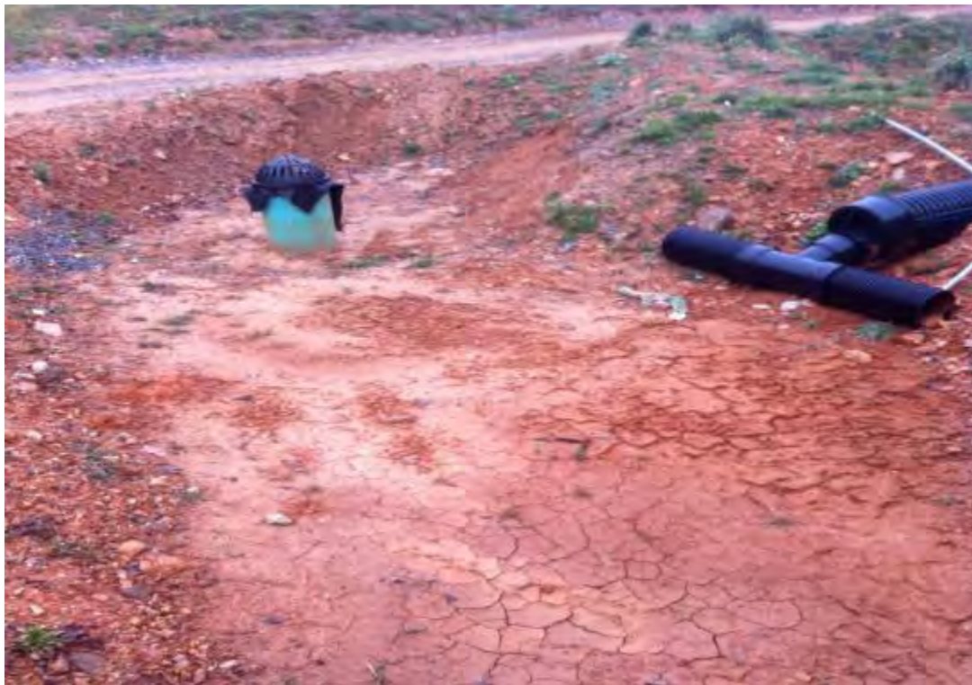
Figure 5.3.4-21. An underdrained bioretention area is used as a sediment trap during construction.
