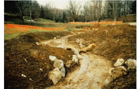
Figure 5.4.1-5. Recreating a meander within a channel, note boulders and curves, and that the right side is higher than the left, which has area for overflow if the water “jumps” the channel banks.
