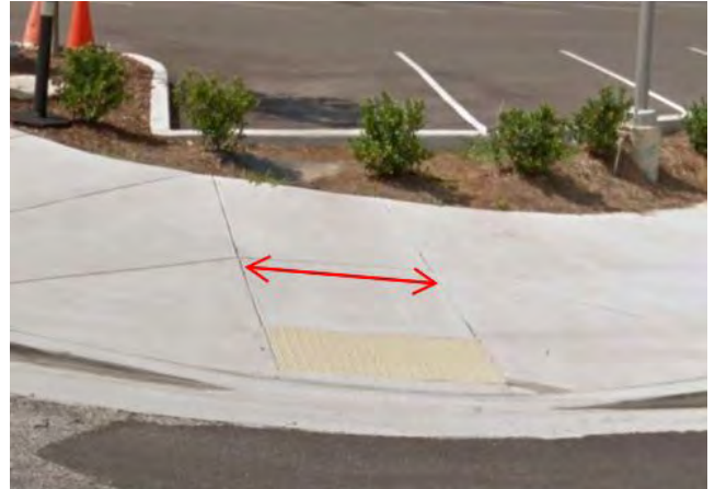
Curb Ramp Cross Slope
