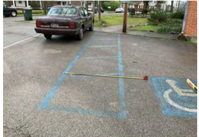
Accessible Parking - Cross Slope in Excess of 2%
