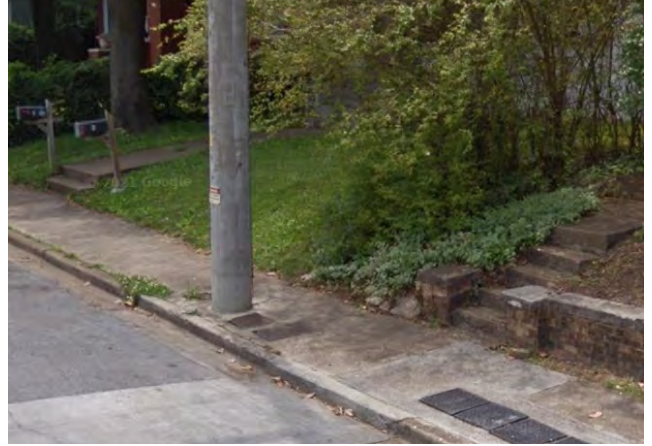
Sidewalk Obstruction – Overhead Vegetation Protrusion
