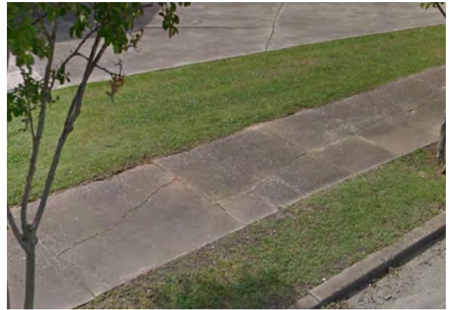
Poor Surface Condition
