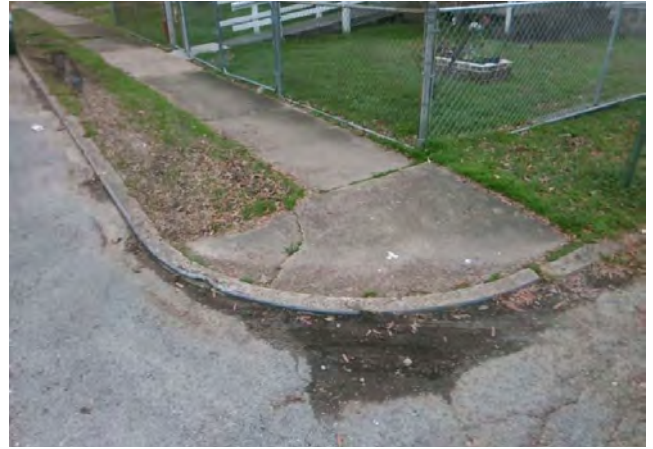
Missing Curb Ramp
