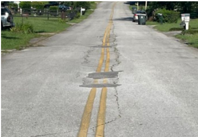
Utility Trench Settlement
