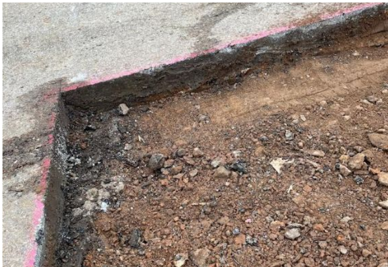
Lack of base
