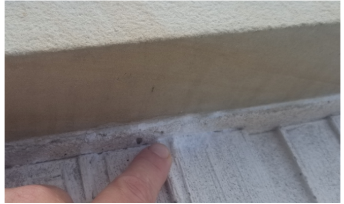
Detail of efflorescence near grout, noted in ~5 areas.
