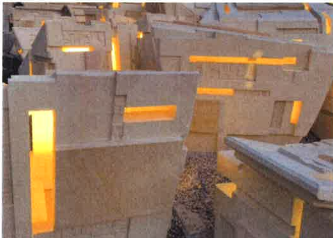
Dusk photo with lights on during Scramble construction in mid December 2020. Vertical 4" wide openings (as shown in the bottom left of the photo) fulfill both aesthetic and technical needs, by providing access to stake mounted light fixtures concealed within the Elements (see more below)
