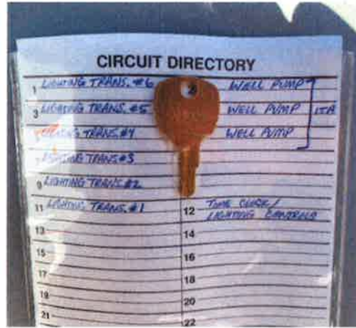
Above: circuit directory and panel key located at panel door interior. Photo during construction in mid December 2020
