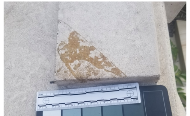
Detail of sticky substance noted on element #14.
