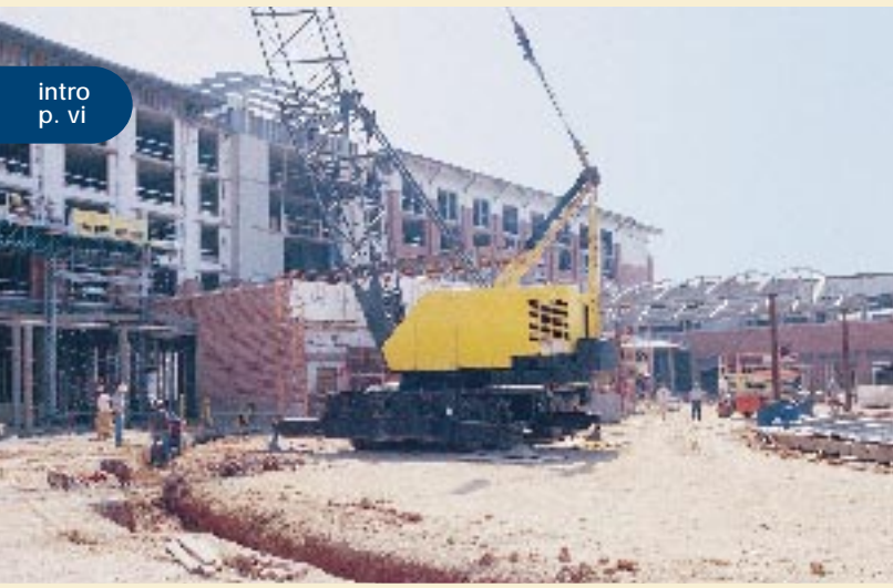
(below) Site of the new Conference and Training Center and the new Parking Facility .
