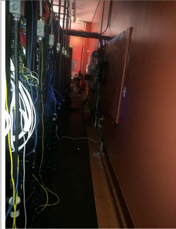
Dangerously inadequate lighting and ventilation in the current data center.
