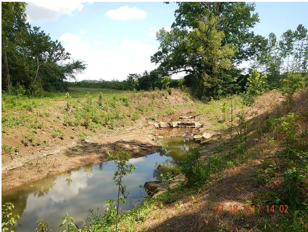
Figure 10 Upstream of bank failure at end of project
