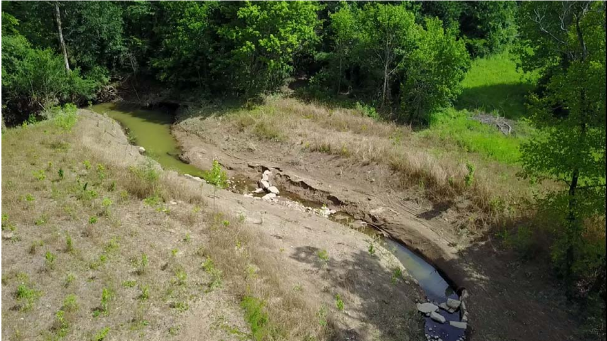
Figure 9 Aerial view of bank failure at end of project
